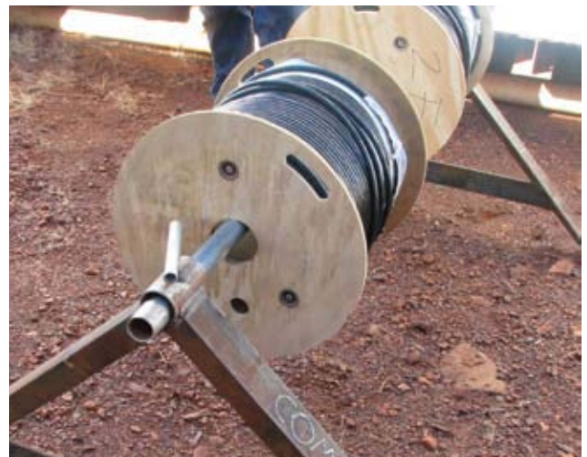
Pre-terminated sacrificial sheath cable is used to prevent termite damage
