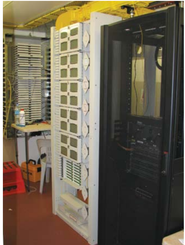
Pre-terminated fibre cables from the FL2000 Distribution Rack connect to the Fibre Entrance Cabinet for splicing to outside plant cables
