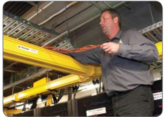
Mike Duffy lays the horizontal cable in the FiberGuide cable management system
