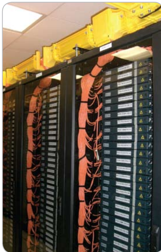
Sliding Fibre Trays with FiberGuide® Cable Management in the Server Room of The Venetian. (Macau Hotel)
