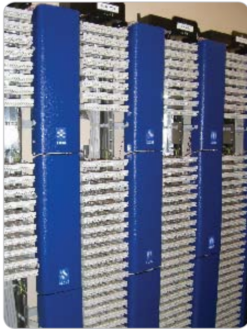
HighBand® 25 Inside The Venetian's Server Room
