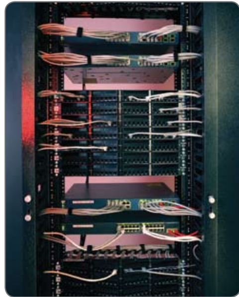
24-port Dynamic Angle Patch Panels direct the patch cords toward cable management on the sides of the rack.
