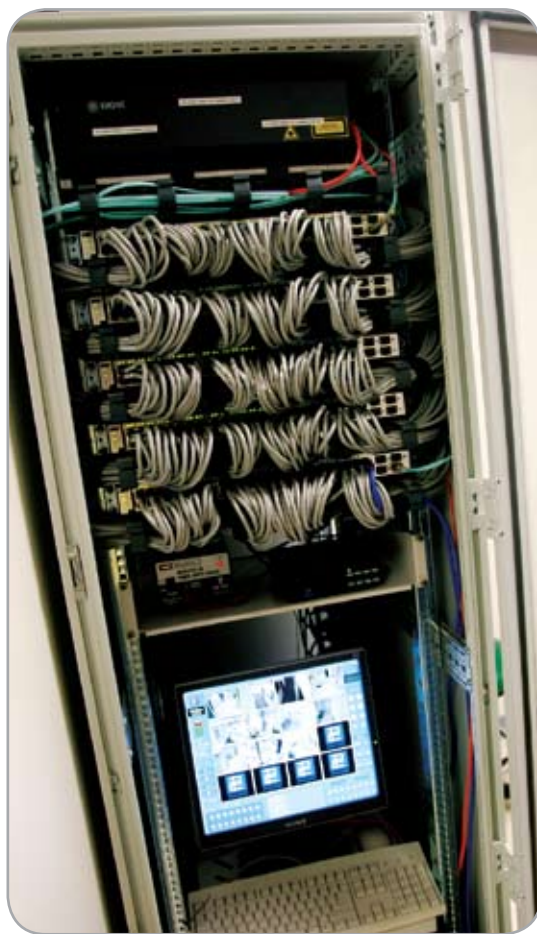
QML's Active Equipment Rack
