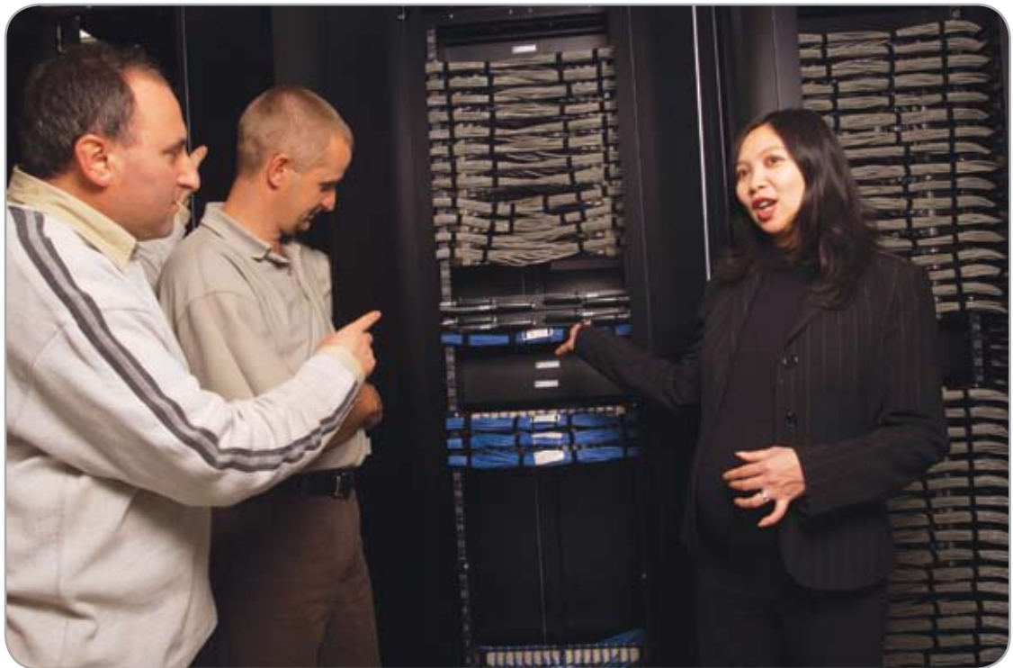
Rear cable management of Optus' Ethernet Distribution Frame (EDF)
