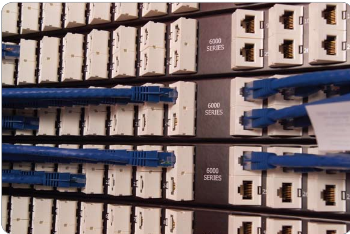
Dynamic Angled Patch Panels
