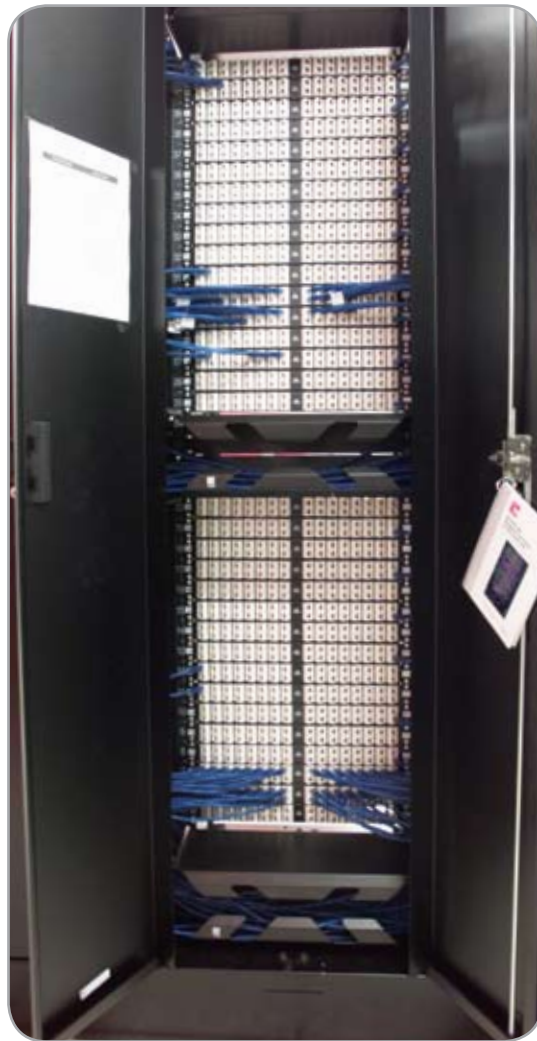
Front Patching area of Optus' EDF
