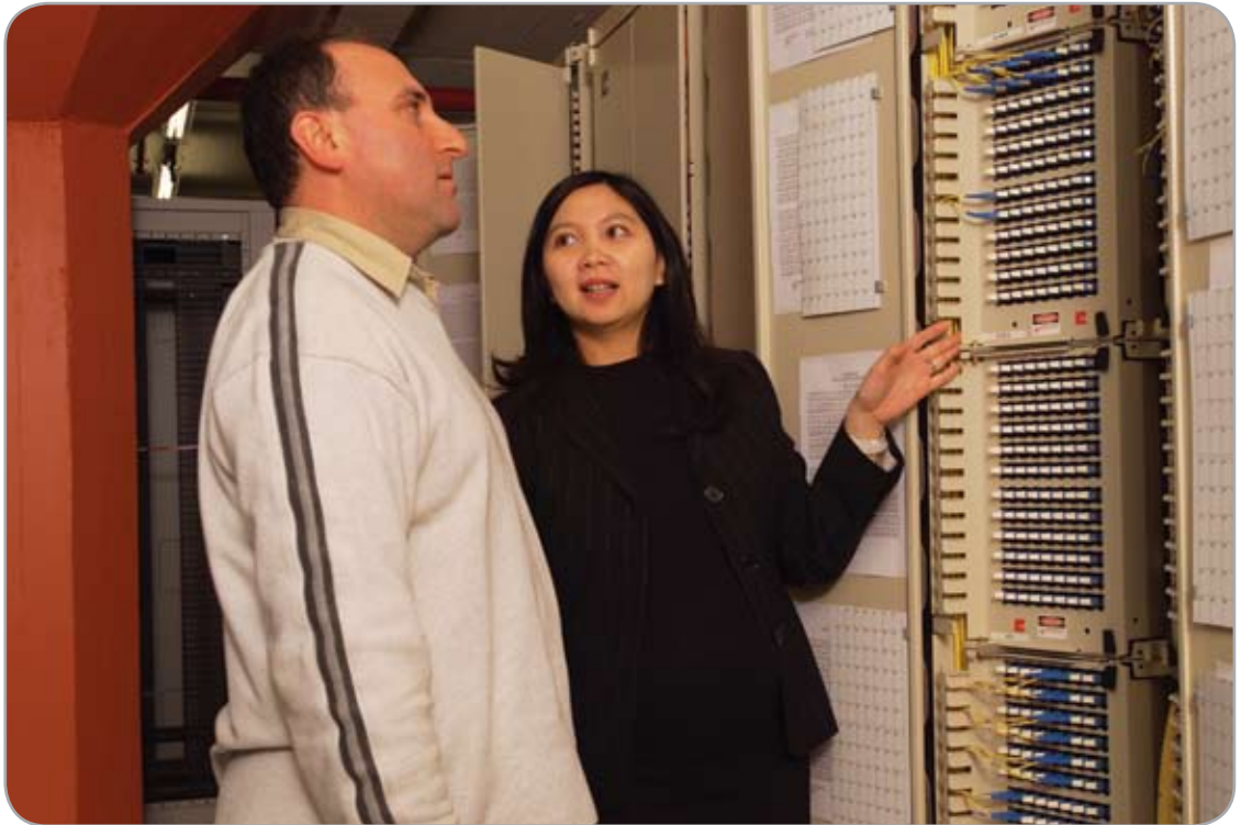
Danny Vertouris, Optus and Adelle Ly, ADC KRONE inspect the OMX-600 fibre distribution frame
