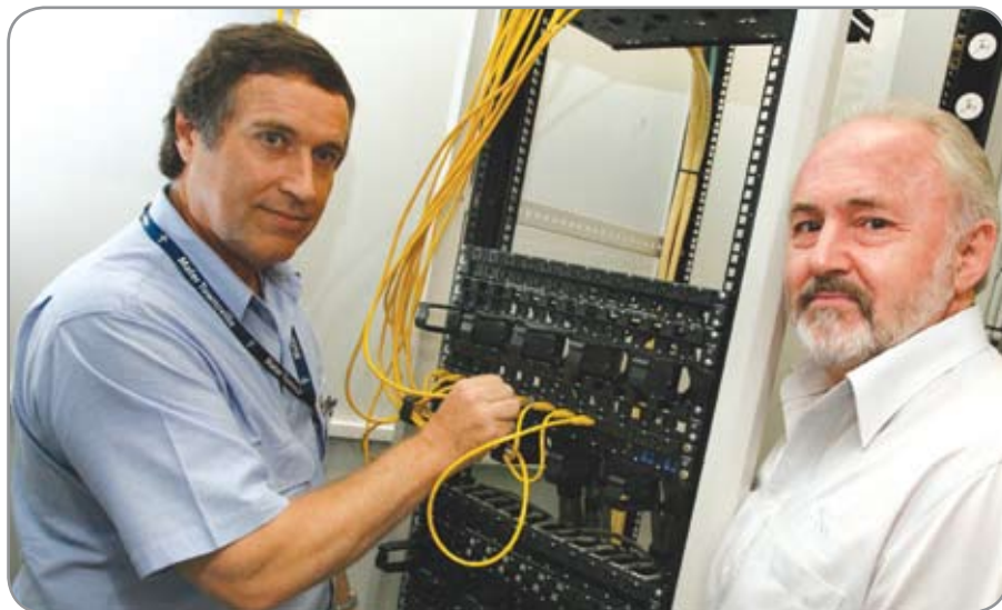
Ian Evans, Mater Hospital (left) and Fred Warwick, PK Business Advantage (right) patch switch ports onto the CopperTen Patch Panel.
