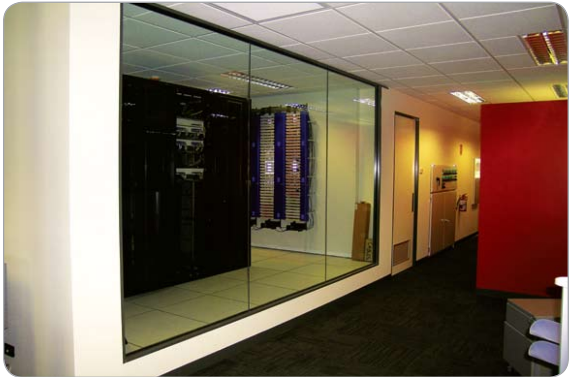
KINCROME's new communication facility
