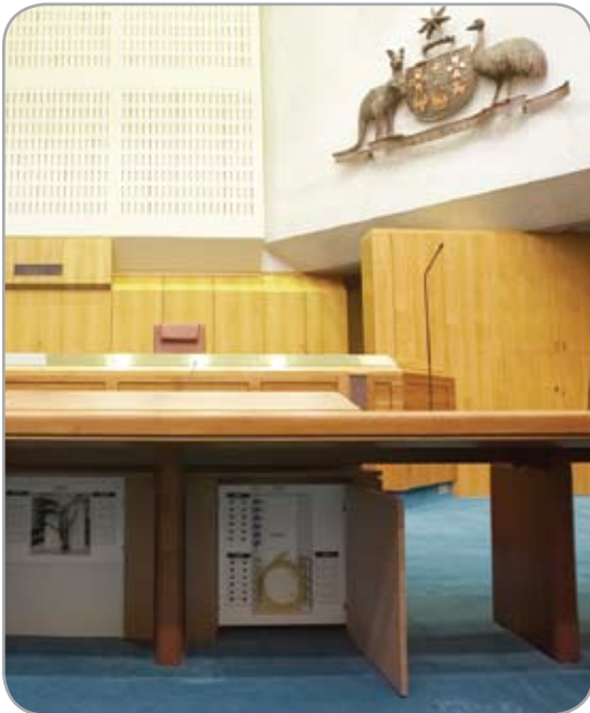
Control and Video Link Cupboard.
