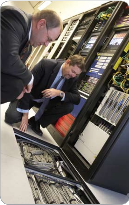
Heath Mackey, High Court and Grant Bawden, Intravision examine the under-floor cabling.
