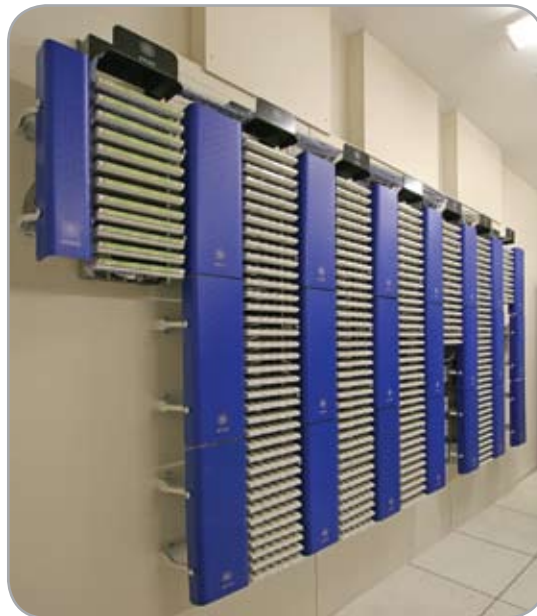
The new HighBand® 25 system in Fisher & Paykel's communications room.
