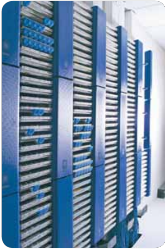
HighBand® frames in the Level 2 communications room.
