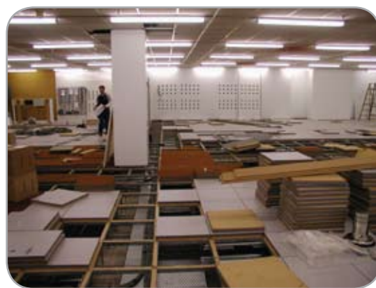
Construction is underway with a false wall for the Profil frames mounted and cable trays installed.
