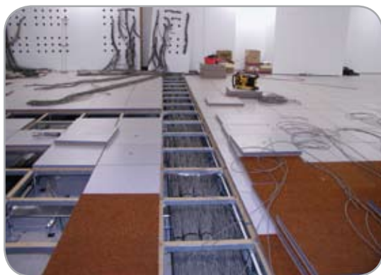
Construction is nearing completion with the majority of Category 6 cables being installed and loomed.
