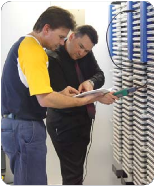
Darren Robertson, Structured Communications, terminates HighBand 25 modules whilst ADC KRONE's Alex Price conducts permanent link testing.
