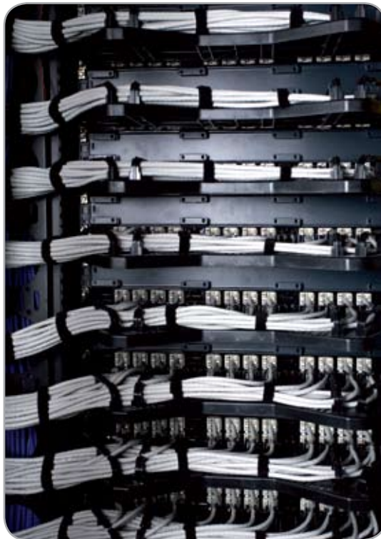
Masterminder Cable at rear of rack.
