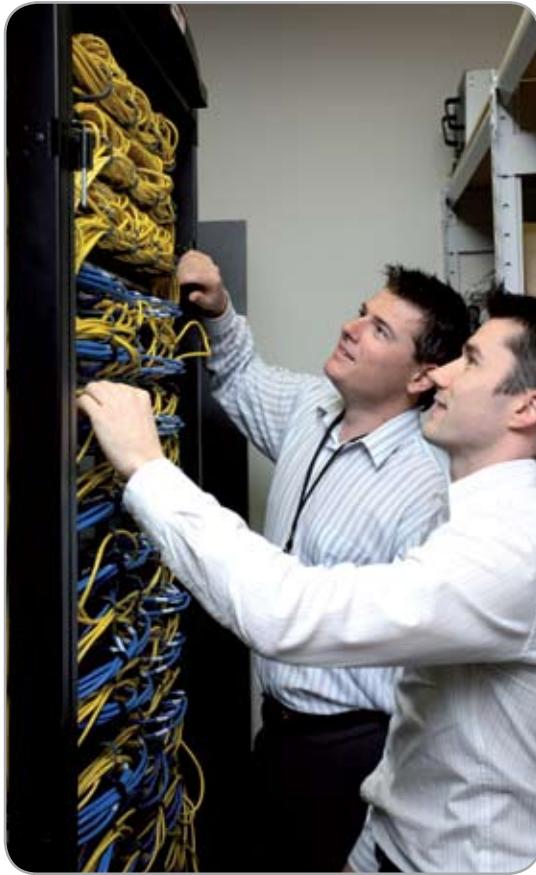
Danny Smith (left) from Cable 8 and Keith Lawrence (right) from Clough examine the setup.
