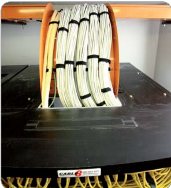
Good cable support at top entry to cabinet.
