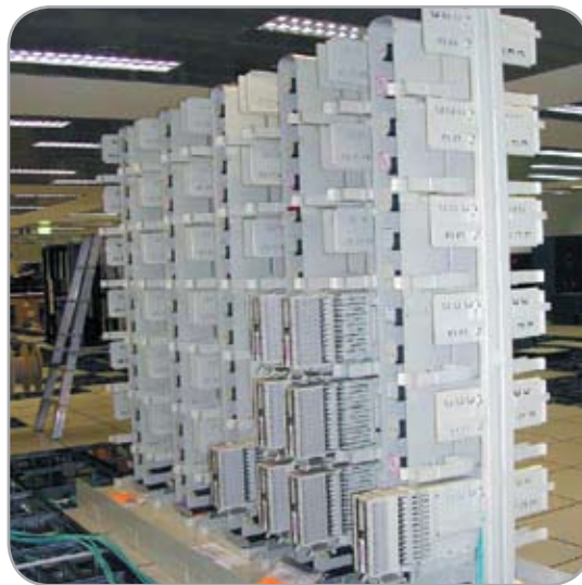
Next Generation Frames are positioned back-to-back to save space and allow easier and more secure routing of fibre between frames
