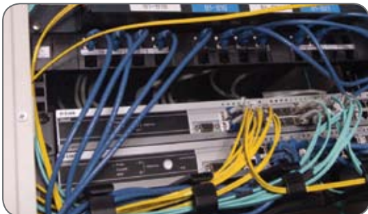
Left: One of the diverse backbone cable entries under the Temple Building
